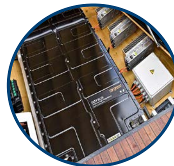
BOAT BATTERY PACK 20 KW/H
