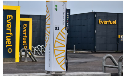
Everfuel hydrogen leakage 2023
